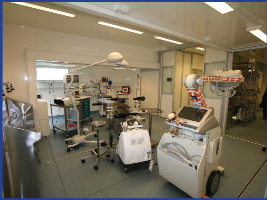
The Operating Theatre also contains a mobile x-ray and ultrasound machines.
